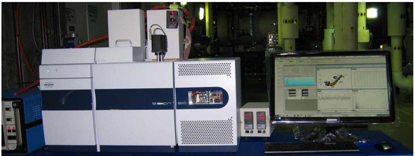
On-line Toxic Organics/Siloxanes in Biomethane Analyzer at an active sewage treatment plant.
